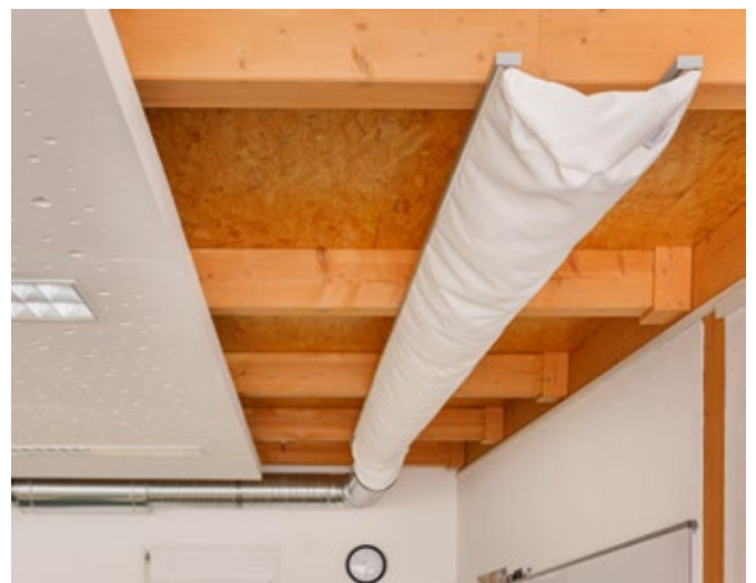
Supply air flows into the room via an air hose
