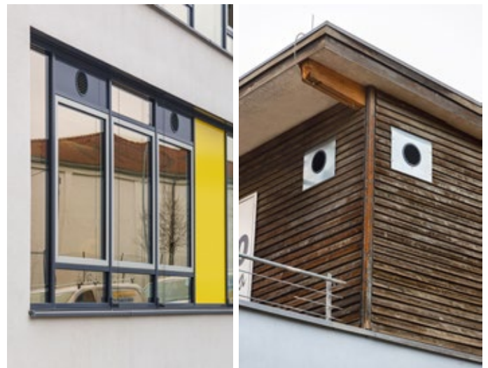
Exhaust air outlets and fresh air inlets are located in the skylights of the windows or at the corner of the outer wall.
