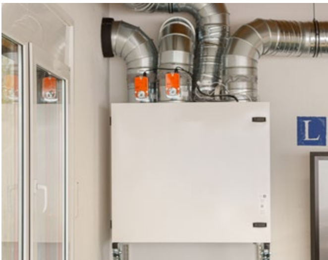
Installation of the Centra ventilation unit on the wall in the classroom, including air ducts & sensor system
